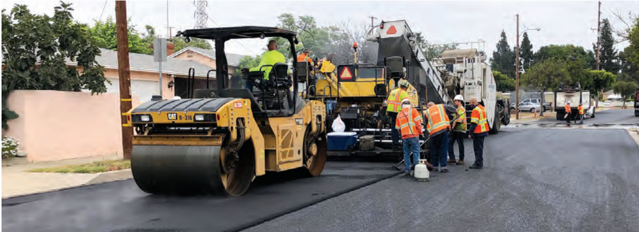
Photo above is the HyRAP® going down onto the paving interlayer ARAM. ARAM is a proven paving strategy that helps mitigate Alligator cracking.
